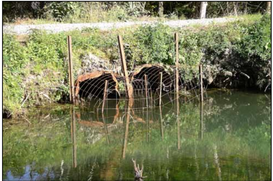
Fencing to deter beavers is one option, but generally is not normal practice for road culvert installation and may require streambed modifications.
