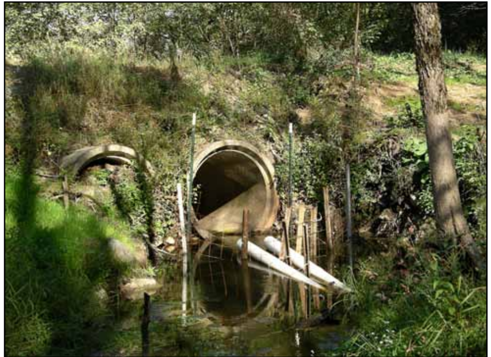
IF&W staff recently attended a workshop on how to prevent beaver damage to road culverts. With new designs in road and culvert construction, efforts to stop beaver damage to roads and habitat are being reviewed and upgraded.
